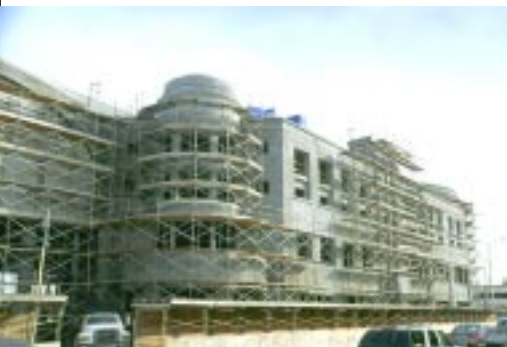
The Shops at Sunset Place is Simon's 510,000 square foot specialty center under construction in South Miami, Florida. This project is scheduled to open in October 1998.
